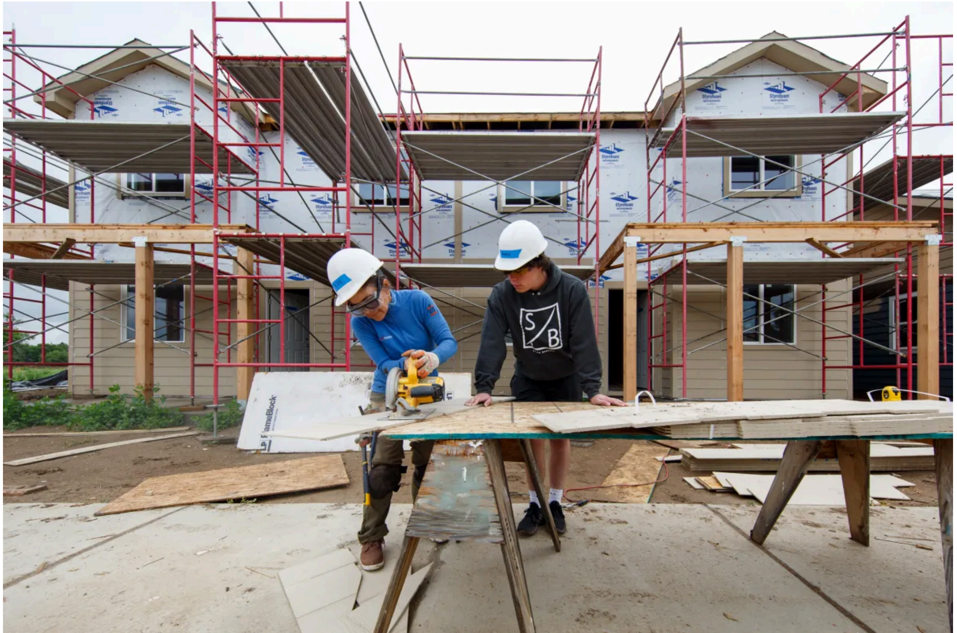
From left, Elen Gaion and Quincy Deibert assist with construction, Friday, June 16, 2023, at VCP Village, a tiny home community for military veterans in Longmont. (Jeremy Sparig, Special to The Colorado Sun)
